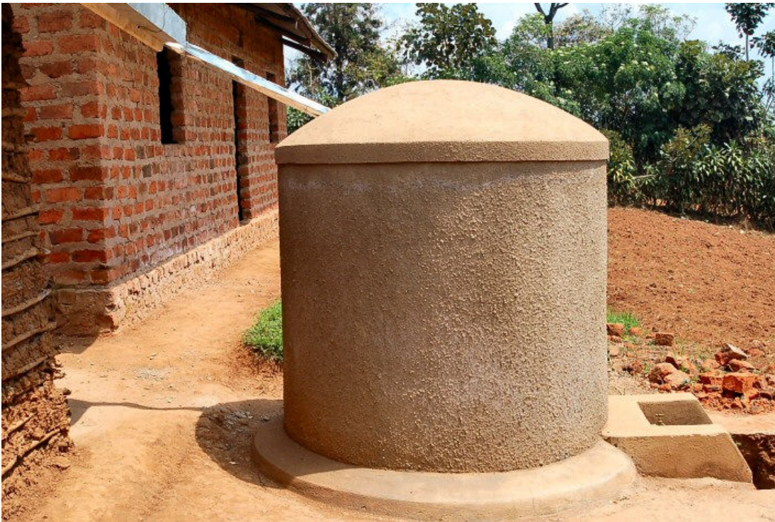
A smaller tank we built for the project, holding 6000L
